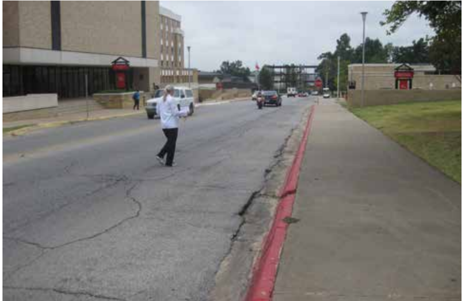
Pedestrian crossing Caraway Road east of the Carl R. Reng Student Union
