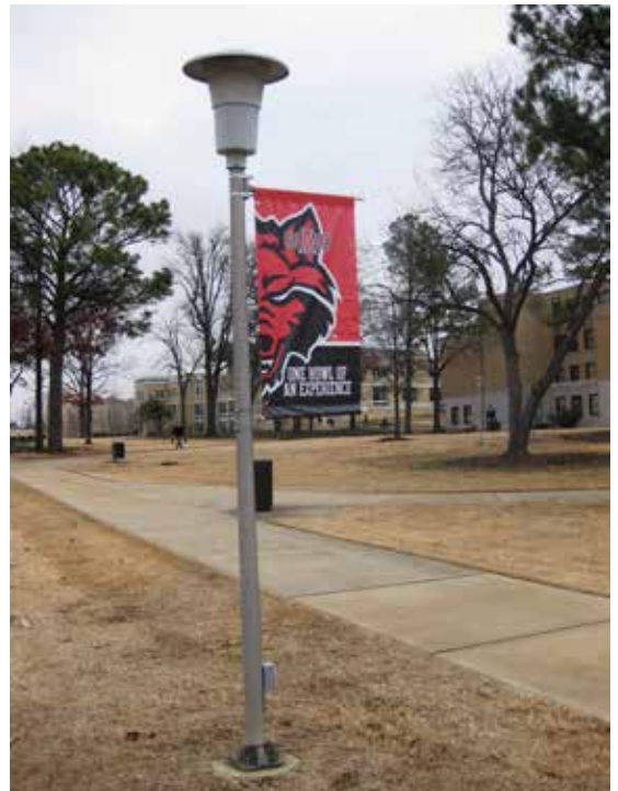
Non-conforming fixture with banner mount attached.
